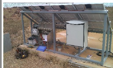
Example of a remote field unit set up incorporating industrial pc, solar panel and battery
